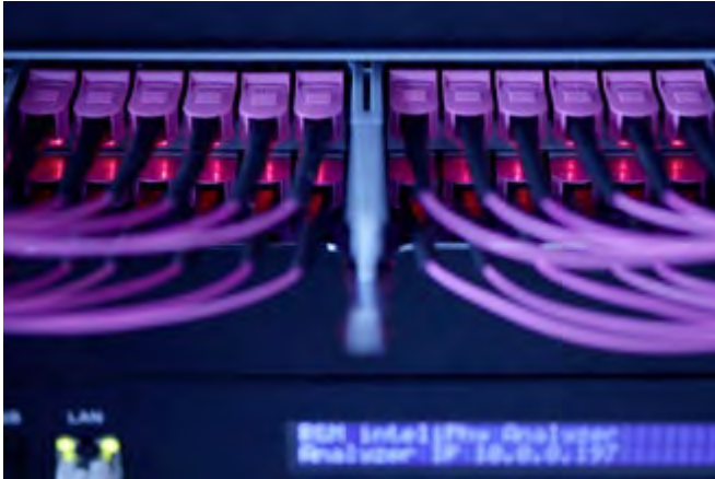
090.7810 R&M inteliPhy of the Netscale platform
