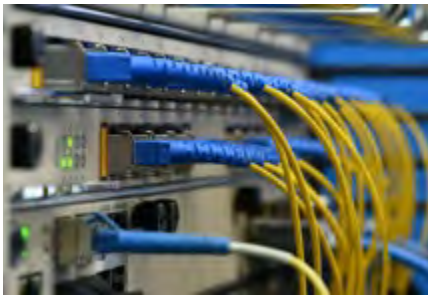
030.6124 Network equipment with singlemode patch cords
